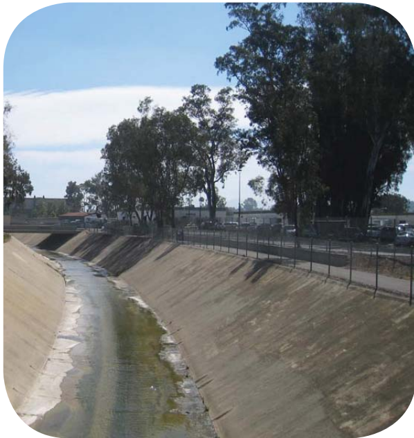
Surveillance Cameras to be Located to Monitor Both Trail and Creek Channel.
