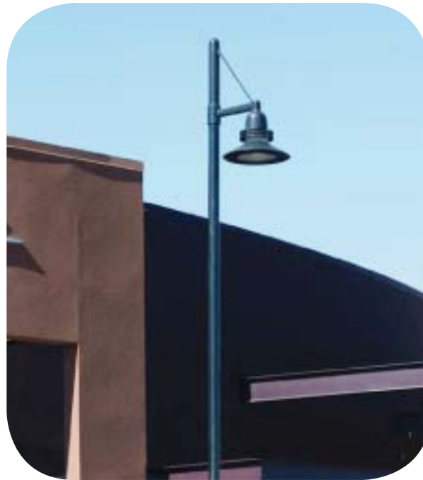
Pedestrian Pole Light with Directional Hood Solar Power Lighting Should Also be Considered.
