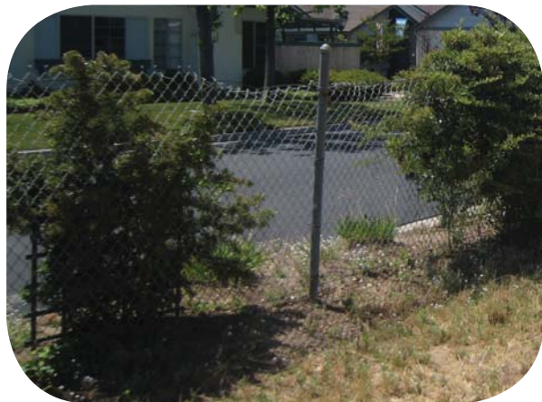
Fence Damaged by People Jumping Fence to Access the Trail
