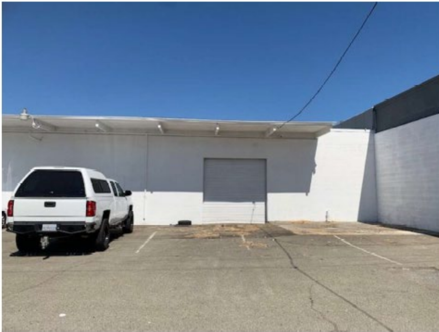
SOUTH SIDE – EXISTING ROLL UP DOOR (TO BE REMOVED AND WALL FILLED IN)
